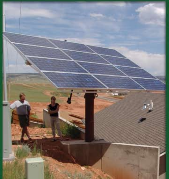
The photovoltaic (solar electricity) system at 2360 Ames Court has a tracker that follows the sun from morning to night. It has a 25-year warranty and can withstand high winds and 60 mph, golf ball-sized hail.
